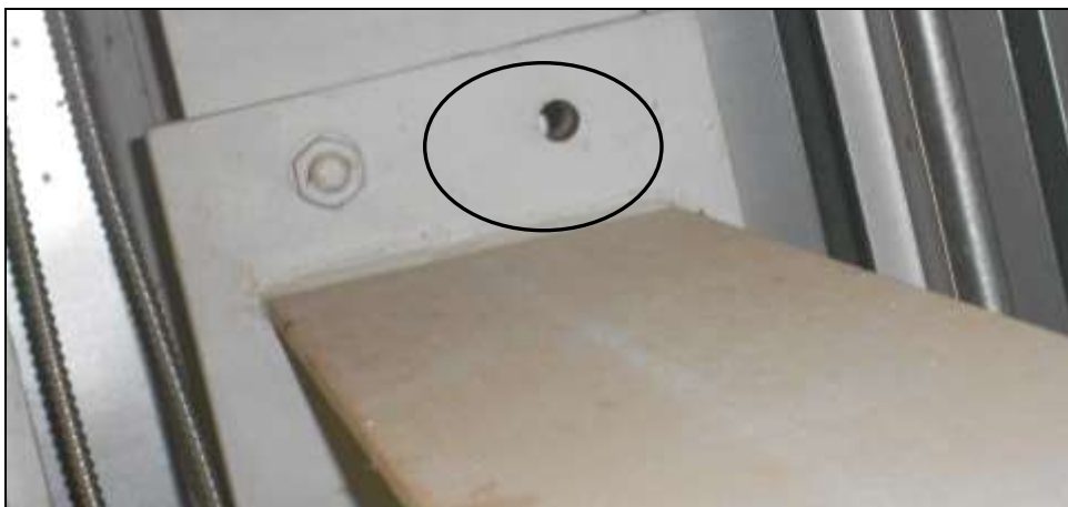
Figure 9 Missing bolt in top plate of the steel column. Add bolt and check all columns or connections to make sure bolts are installed and torqued to manufacturers or installation specifications.
