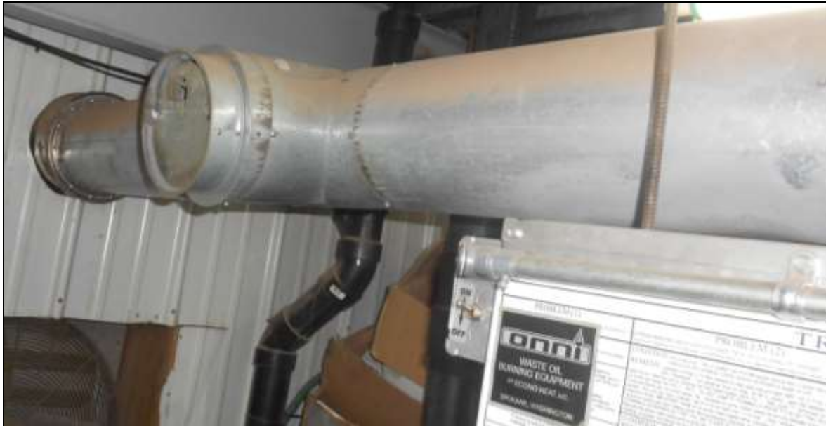
Figure 7 Vent connector was too flat; recommend a proper pitch for drafting.
