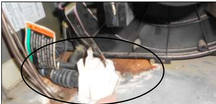
Figure 8 Corrosion or rust inside cabinet; have an HVAC contractor evaluate and service system.
