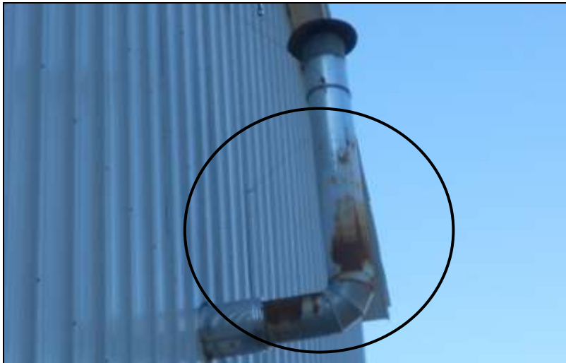
Figure 5 Metal chimney for the Omni waste oil burner was corroded. Have a chimney contractor evaluate. Vent connector off the furnace had heat/scorch marks and soot.
