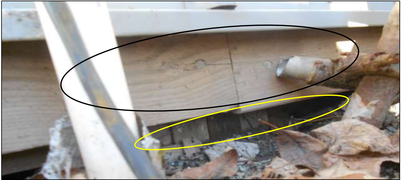
Figure 10 Wood 2x4s facing out and several (7+) nailed together perpendicular to the front 2x4. There was siding overhang approximately 2-3 inches where randomly checked in between storage against building. Check the building plans for the siding overhang and wood used under doors or perimeter.
