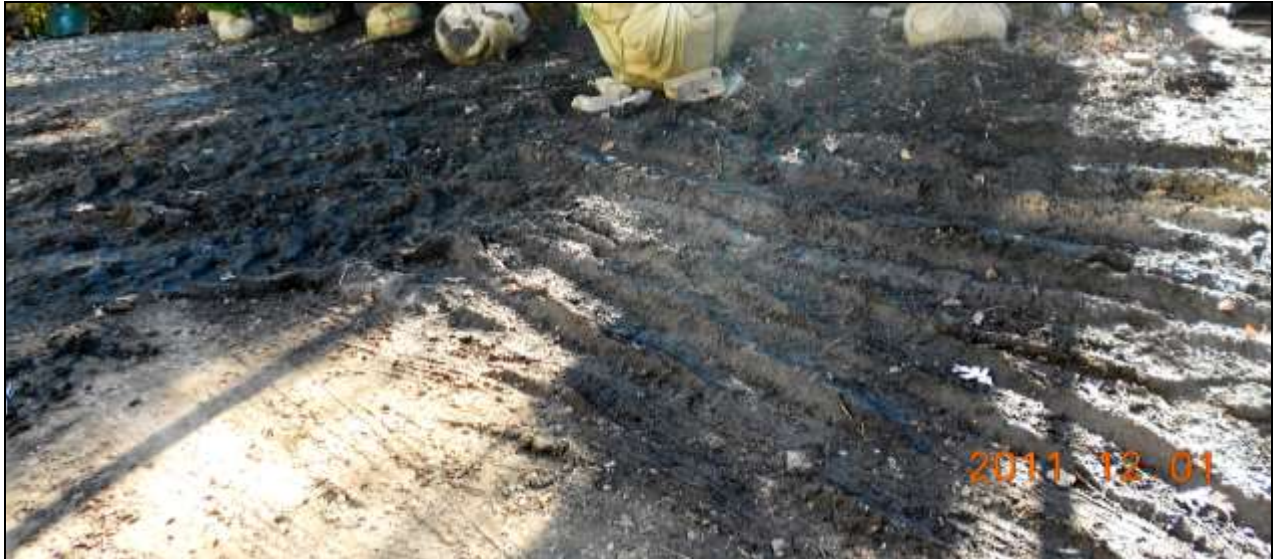
Figure 3 Thick wet mud or ruts around property from vehicles and poor drainage. Recommend stone, gravel or asphalt where for vehicular traffic. Drainage needs to be corrected; confer with a drainage/soils contractor or engineer.
